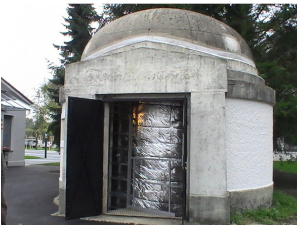
Fig.2. Main storage tank at district heating plant in Graz, Austria
