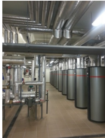
Fig.3. Heat pumps used as auxiliary heat sources in a heating plant in Katowice, Poland
